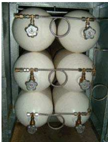
Natural gas storage unit at a BONSAI refuelling station
