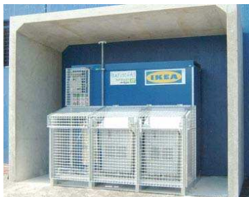
BONSAI natural gas refuelling station
